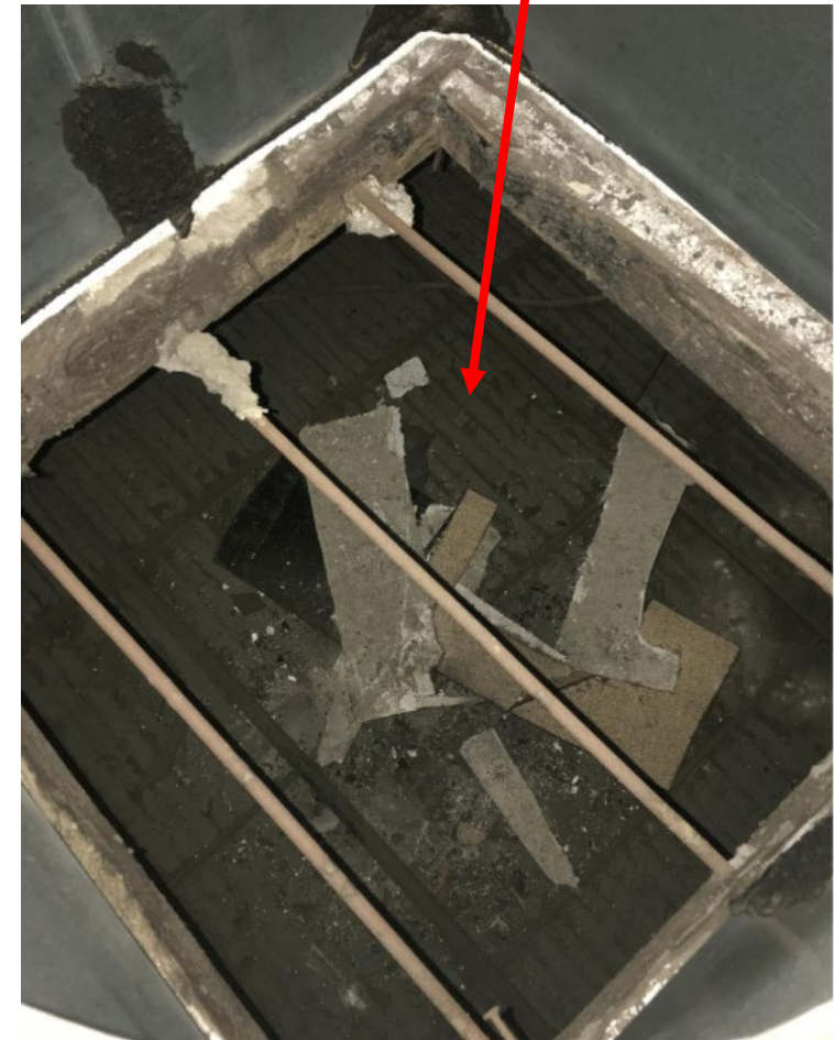
~2ft Cavity with No Insulation
