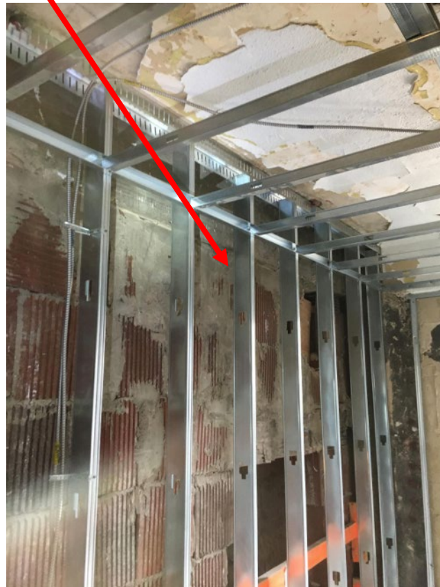
GAP between stud and masonry
